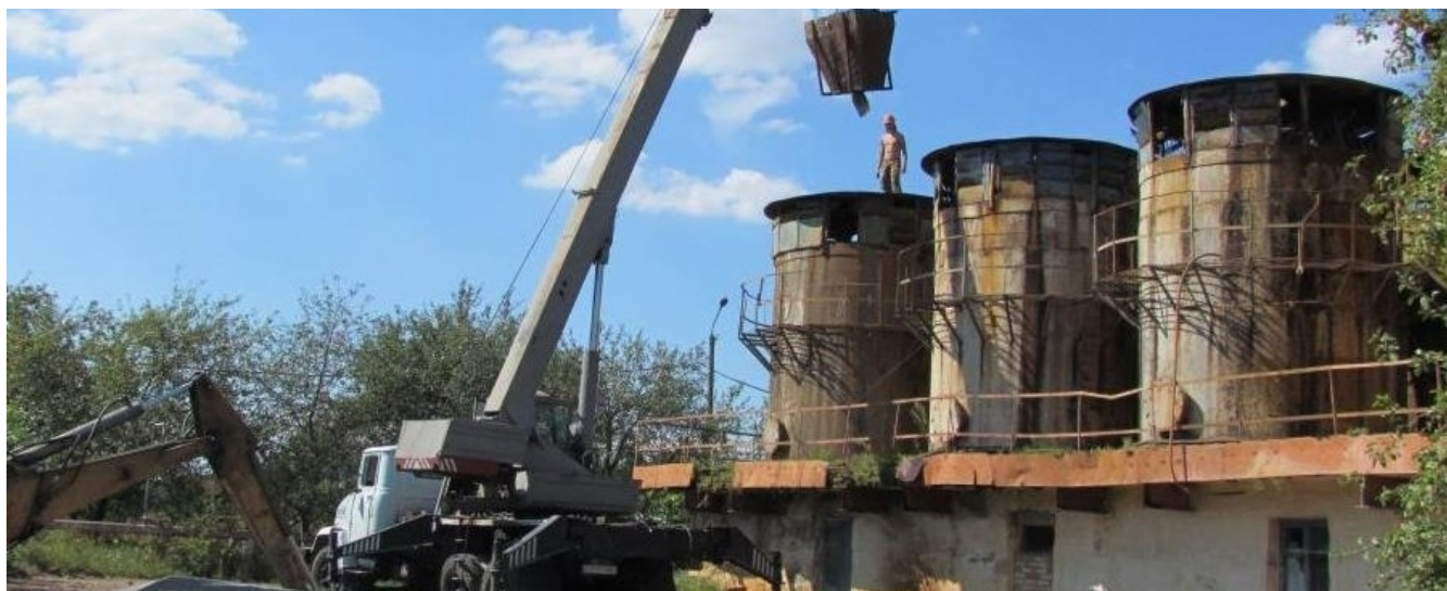
Fig.3.2 Iron removal system in Fastov
