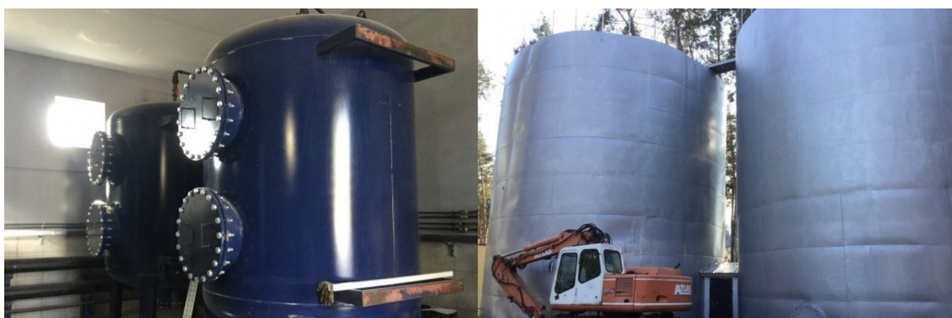
Fig.3.3 Station of deferrization of water of Irpen Vodokanal
