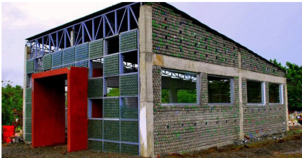
Fig. 3. A school in the Philippines made of old plastic bottles filled with adobe [22]
