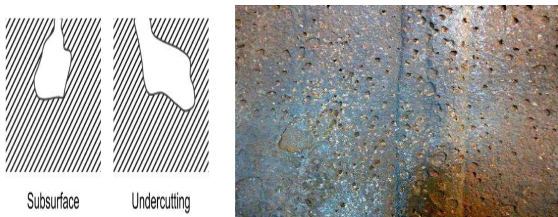
Fig.1.13 - Pitting corrosion: a- profiles of the pitting corrosion; b – surface of the metal damaged by the pitting corrosion
