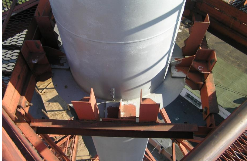
Figure 1.11 Horizontal load transfer unit using sliding supports: a) design of the horizontal load transmission unit; b) a node for transmitting wind load from the pipe to the tower.
