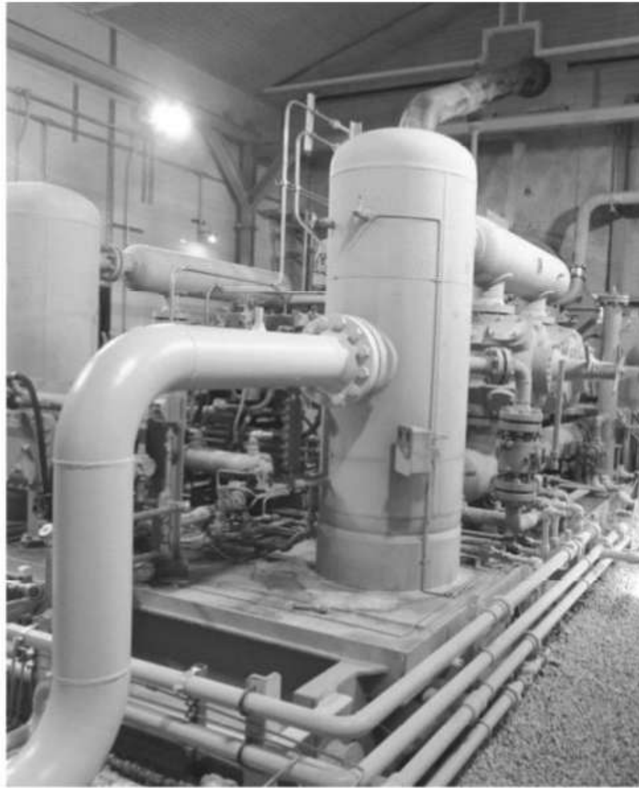
Figure 2.1- Inside compressor building.
