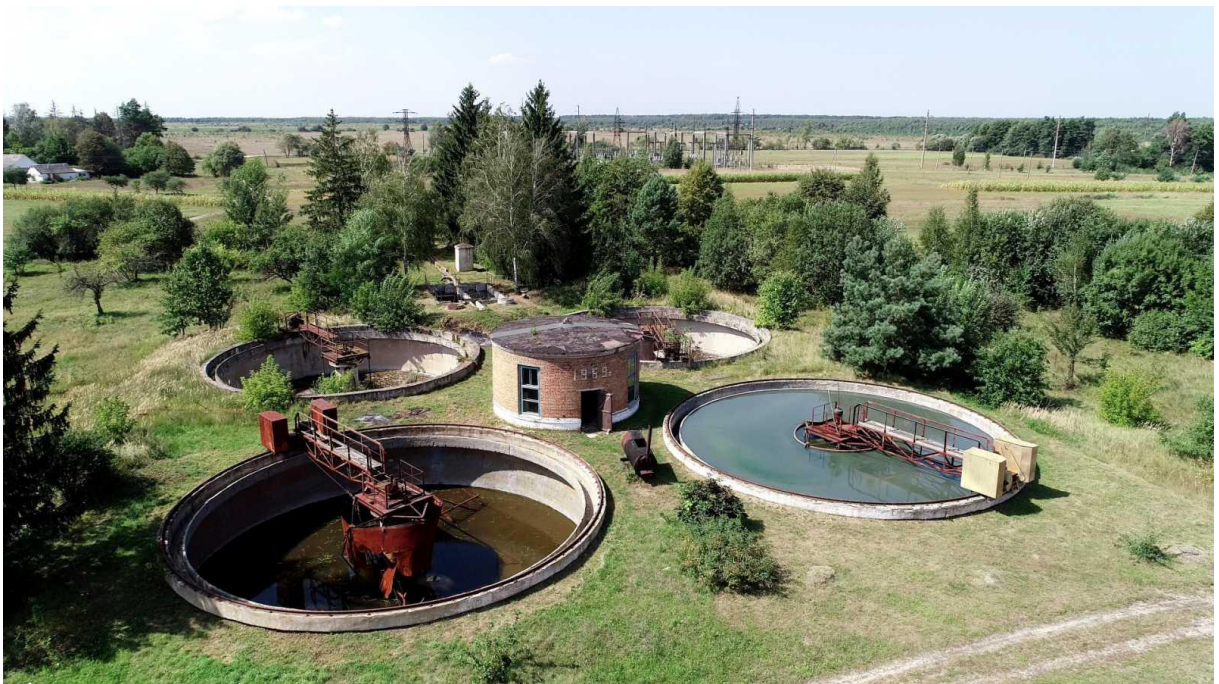
Fig.1. Current state of defunct sewage treatment plants
