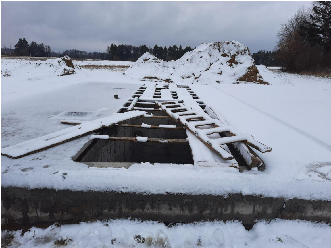
Fig.8. Completion of the construction of the underground part of the structure (winter 2022)
