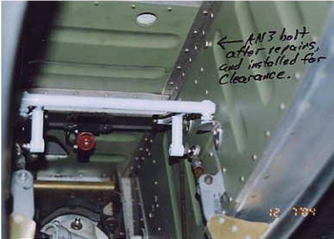
Right nacelle the wire breaks corrosion of terminals hinges
