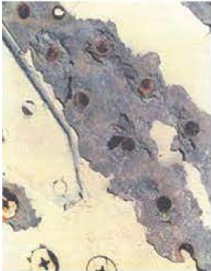
Galvanic corrosion between magnesium surface and steel connections
